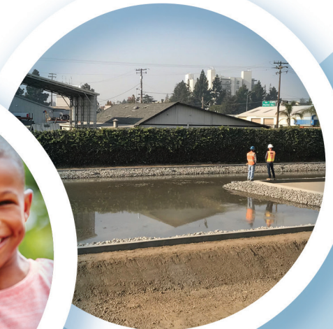
Gish station's system for retention of well flushing water
